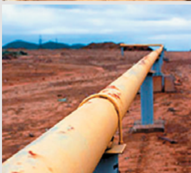
West African Gas Pipeline.
